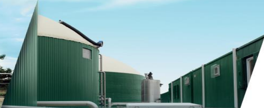
SOUTH MILFORD (UK) - 530 Sm 3 /h BM and 500kW Waste pre-treatment and BTS Upgrading System Organic Waste
